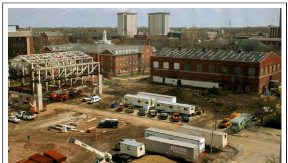
Rising northeast of Hamilton and Whitten halls is the bridge over University Street that will connect the two structures that will comprise the Student Fitness and Kinesiology/Recreation Building. McCormick Hall is on the right. The target date for opening the new building is January 2011.
