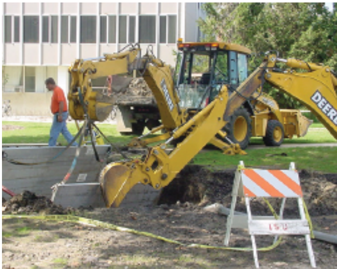
Facilities Management employees Tuesday did emergency repairs to a water line that serves Feeney Dining Service and south campus residence halls.
